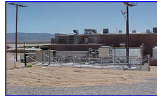
7.5 MW CHP , Twenty-nine Palms, CA
