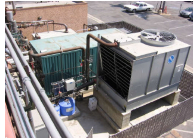
Packaged Combined Cooling, Heating and Power System
